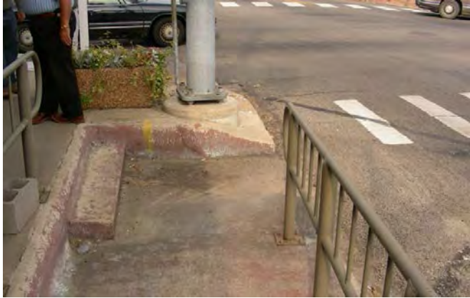
Poor Accessibility (before picture)
