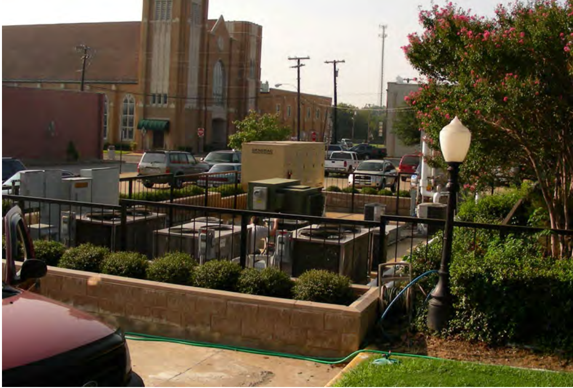
Utility Pad for the Courthouse Located on a Concrete Pad in the Square (before picture)
