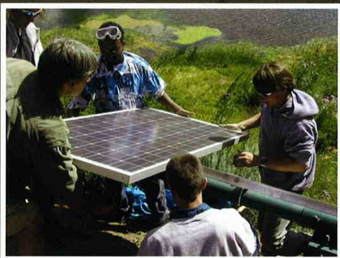
Participants of a Solar Energy International (SEI) class learn how to install Photovoltaic panels
