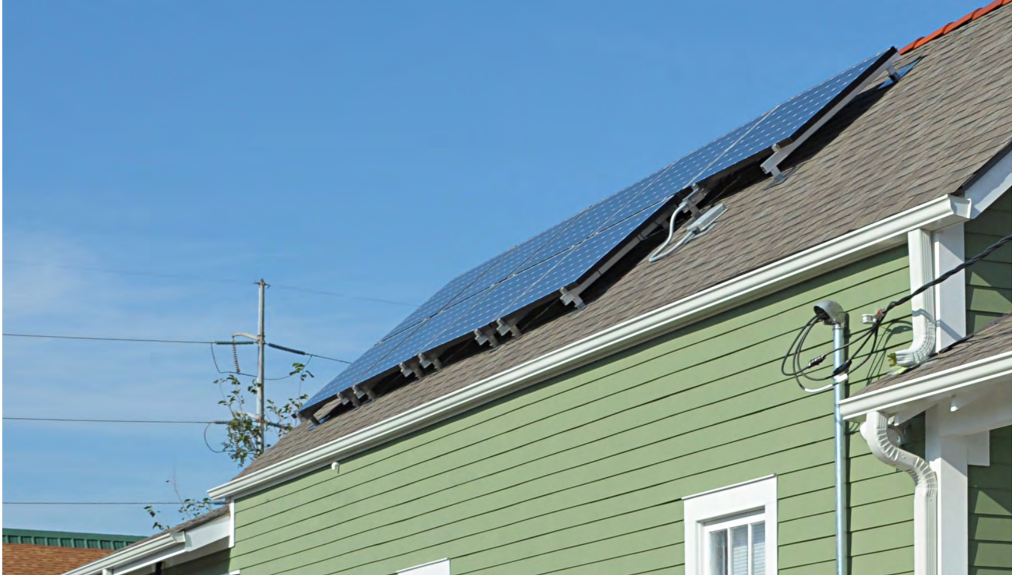
SOLAR PANEL @ 8522-8524 PLUM ST
