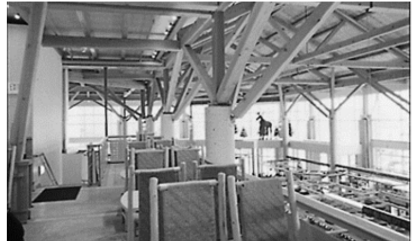
The Douglas fir timber trusses and rafters sit on concrete columns, and were placed by the Timber Framers Guild.
