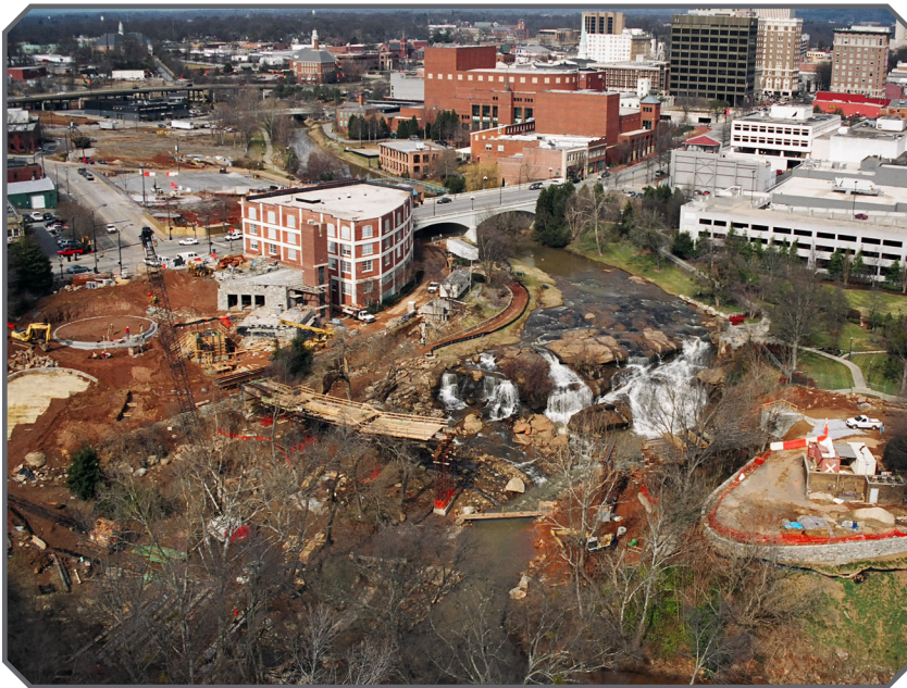
Aerial shot of construction of Liberty Bridge in 2001, photo credit: City of Greenville
