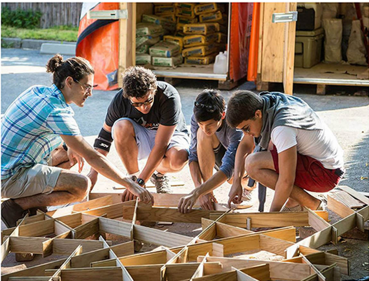
Laying out the trellis with oak floor boards resued from the trash
