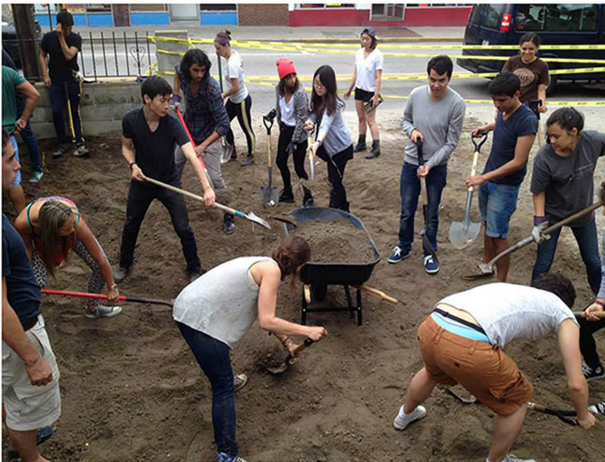
Work begins (all work on the project was done by hand due to extremely limited resources)
