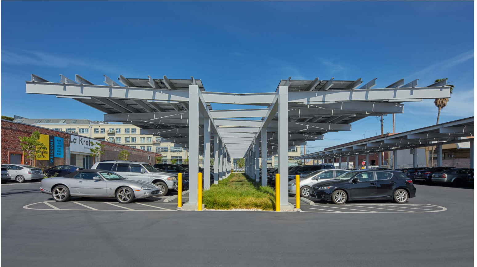
175KW PHOTO VOLTAIC SYSTEM ATOP STEEL SHADE STRUCTURE OVER PARKING
