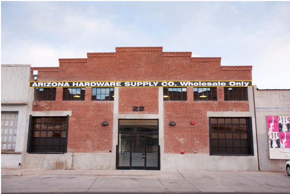
Exterior view at completion of full restoration. The stucco was removed to expose the original brick and concrete framing, the Flemish gable parapet was replicated, original signage repainted, original steel awning windows retained, and new windows/doors installed on façade.
