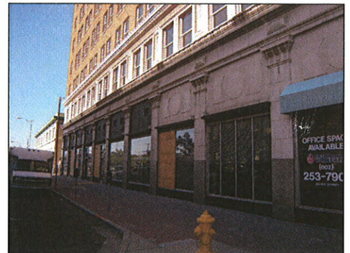
Modern concrete panels in the process of being removed to expose original transom storefront windows.
