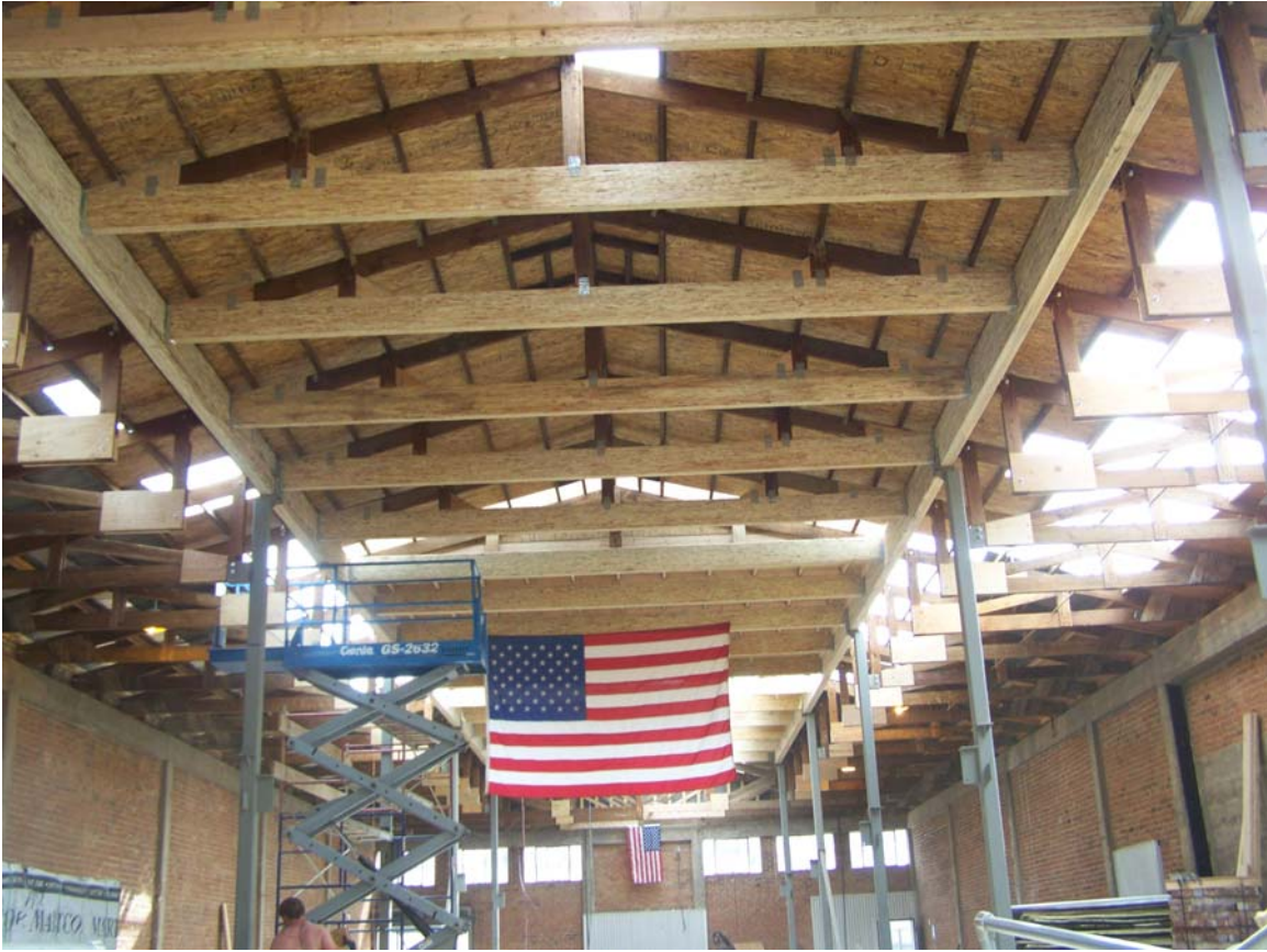
Interior space during construction. New center portion of roof trusses are in place, clearly differentiated as new components, yet structurally integrated with original framing to create a hybrid structural truss that supports roof.
