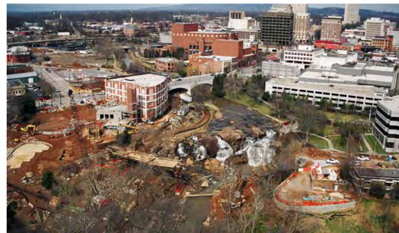
Vision plans completed in 1999 (top) led to the demolition of the Camperdown Bridge in 2002.
