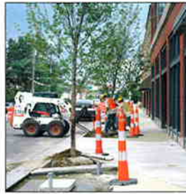
Streetscape construction on the north side of Detroit Avenue is nearing completion.
