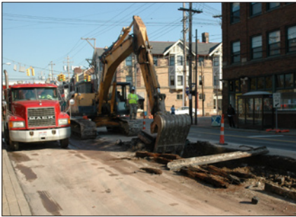
Streetscape construction is underway to transform Detroit Avenue into a pedestrian-friendly destination. The projected completion date is October 2009.
