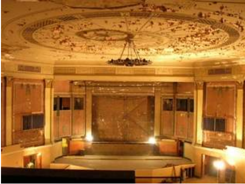
The 87-year-old Capitol Theater in Cleveland is undergoing a $5-million renovation with the help of $1 million in low-interest and forgivable loans from the city.
