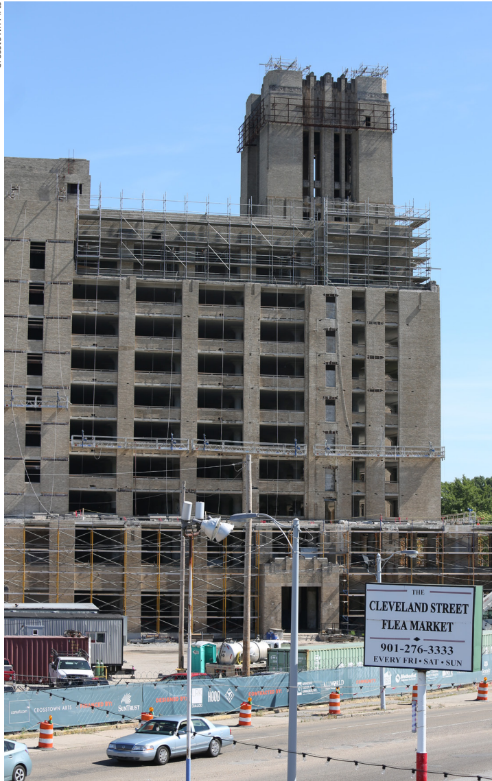
Construction began in 2015 and included extensive community outreach to recruit local contractors and workers.
